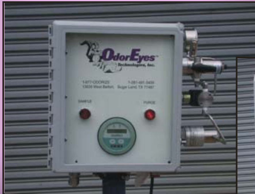
Fixed OdorEyes Monitor System
